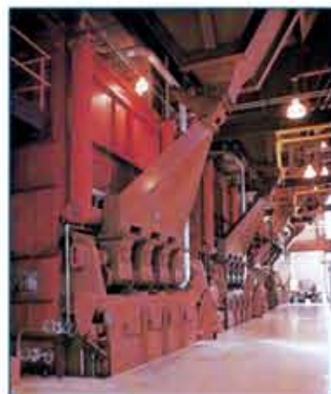
• Solid Fuel LaMont's in a District Heating Plant •
