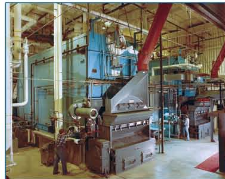
• 2 VL's installed in a heating plant •
