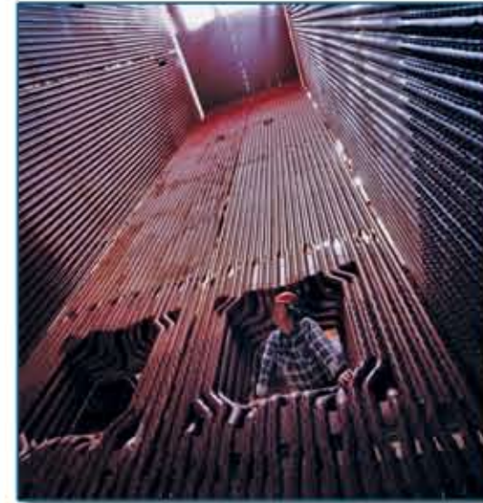
• Membrane wall furnace with two burner openings in an RDF fired boiler •
