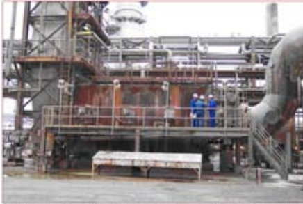
Superheated waste heat recovery Keystone 'O' boiler and economizer after 25 years of service
